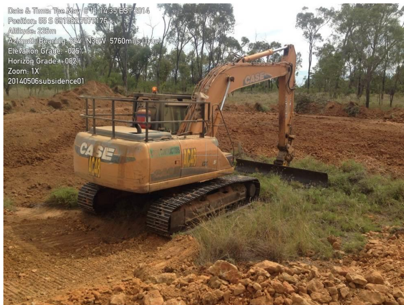
Figure 3 – Excavation of Topsoil from significant cracks
